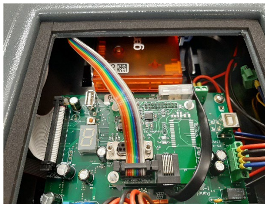
Figure 15: installed modem in the I-SAFE housing
