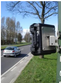
Figure 9: radar installed on the pole bracket
