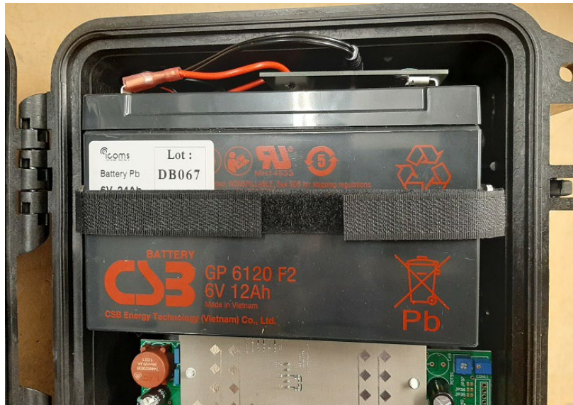
Figure 31: battery placed in the housing
